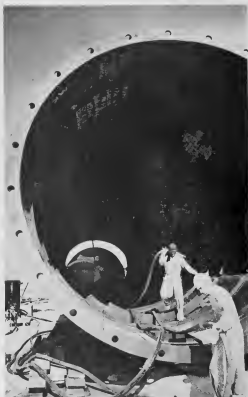
INTO THE cavernous mouth of a furnace stack section go sandblasters, shielded with masks and protective clothing. Taken down to bright metal, the stack's surfaces will be treated with corrosive-resistant materials.
